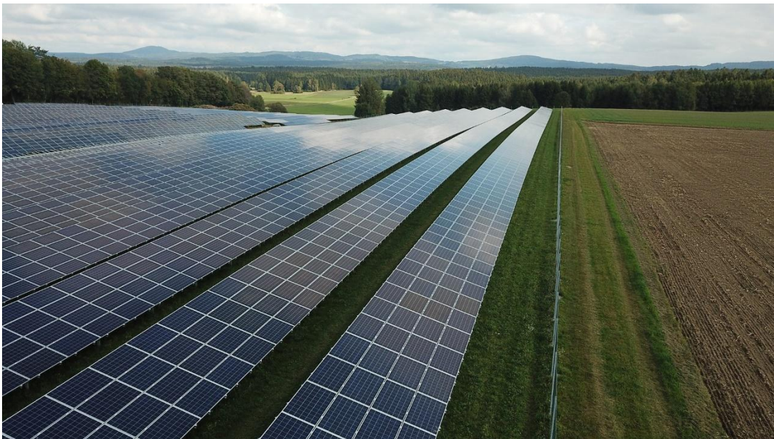
Figure 11 - Photovoltaic Panels - Free picture
